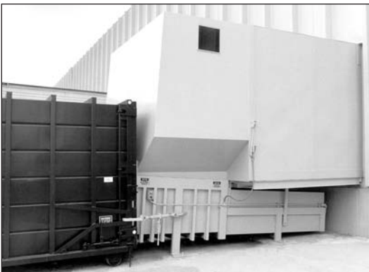
Fully Enclosed Dock Installation
