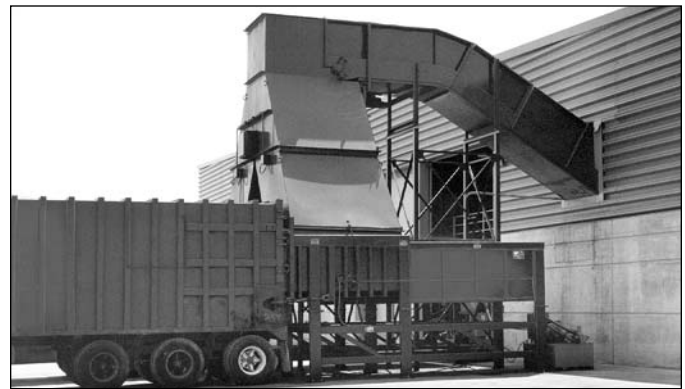
MRF (Material Recovery Facility) Installation
